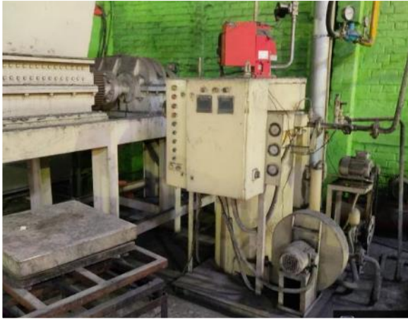
Incinerators installed for BMW disposal
