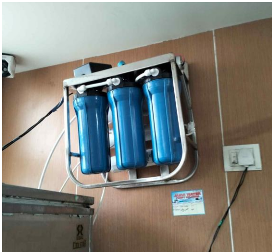
RO for water filtration
